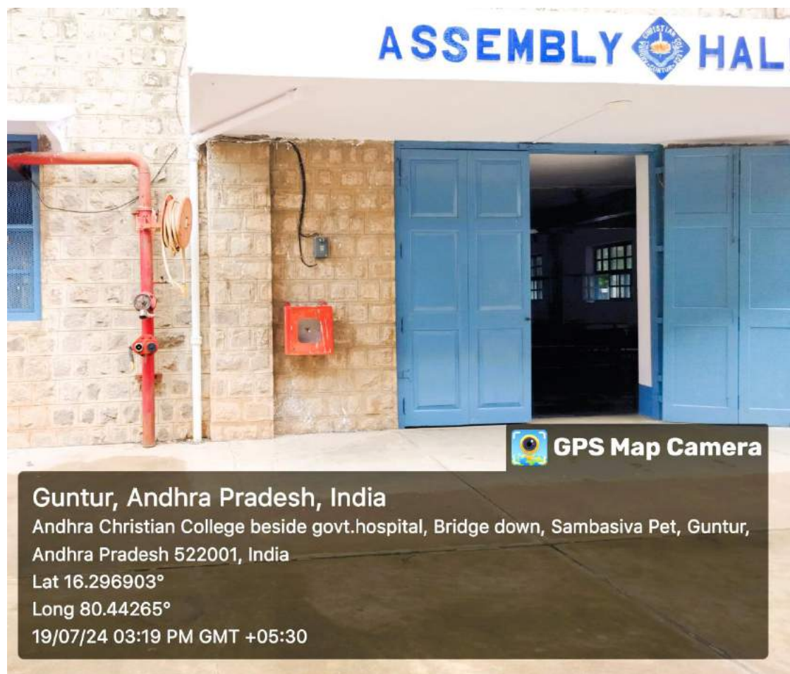
Fire – extinguishing system and Hydrant Valve
